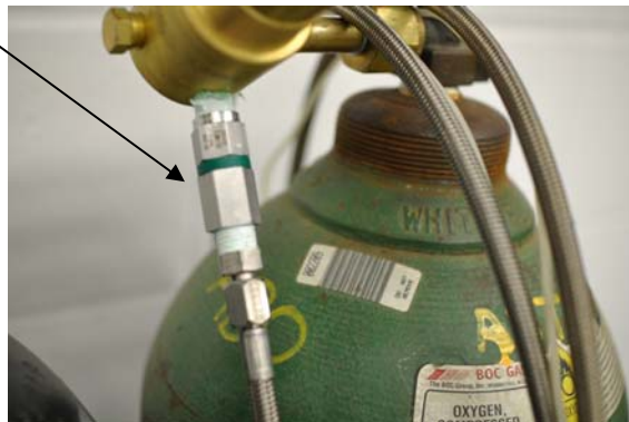
Excessive Flow Valve (Included with 2013 Models. Factory Recommended for Retrofit on 2005 Models)
